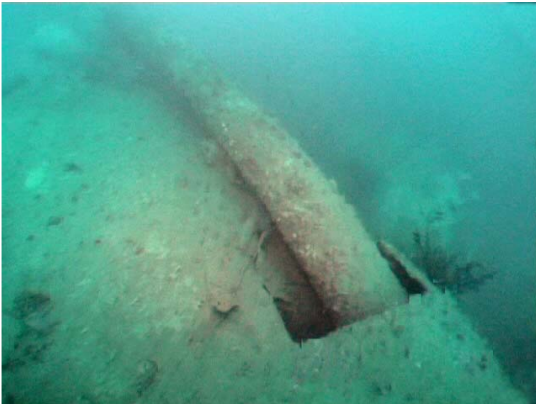
X1/1- Only slight deformation is visible under the outer Starboard shaft at hull exit point.
